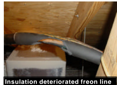
Insulation deteriorated freon line
